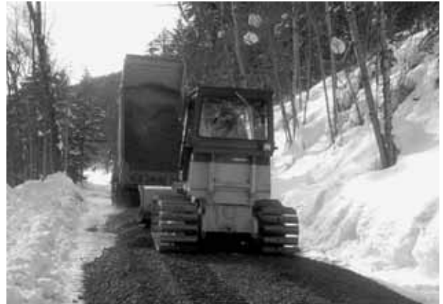
Figure 3 Maintenance (Gravels are supplied for the surface of pavement. The average volume of gravels is about 0.49 m 3 /m.)
