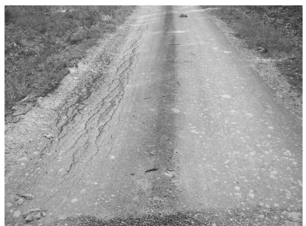
Fig. 13 Left rutting on Finnish asphalt (Ver. 8)
